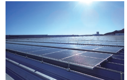
Saitama Factory Automobile Plant (2.0 MW)
